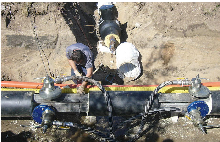
Line Stopping DN125 with connected by-pass for uninterrupted connection of a new pipe line.
